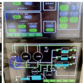
System control panel
